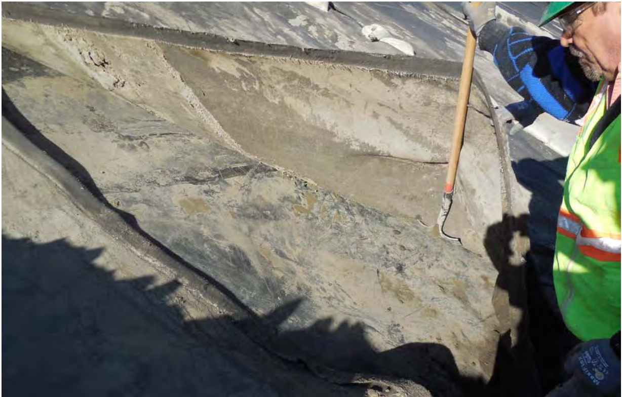
Photo 8 - The liner surface was inspected to confirm that the liner was undamaged.
