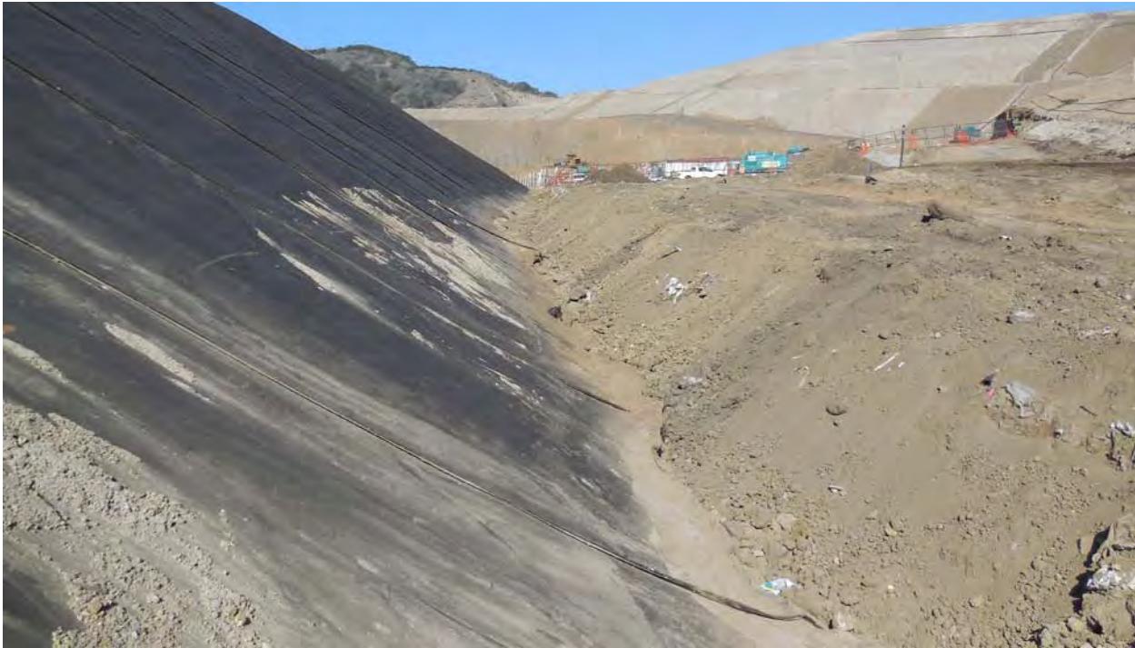
Photo 1 - The area was covered with daily cover soil prior to the cleanup and repair work.
