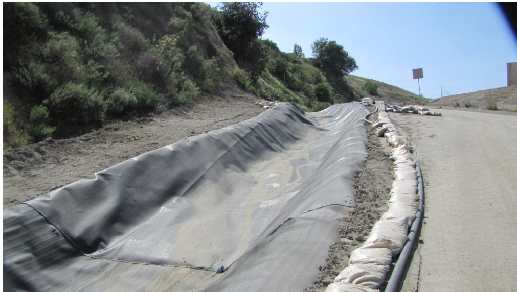
Figure 1 – Interim Drainage Below Scalehouse Area – Damaged liner removed, channel graded and new 60-mil liner material installed
