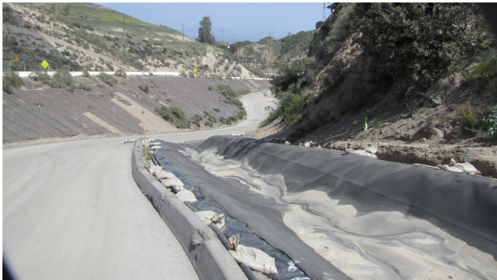
Figure 2 – Interim Drainage Below Scalehouse Area = Damaged liner removed, channel graded and new 60-mil liner material installed
