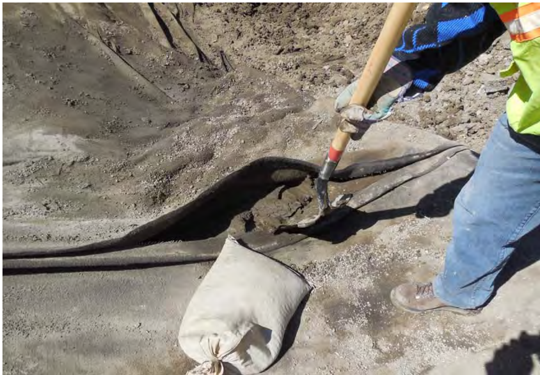
Photo 4 - Fine-grained soils were observed under the geotextile.
