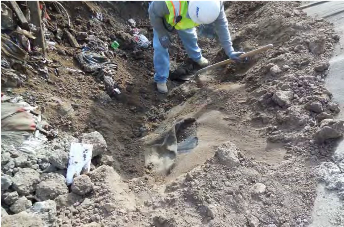
Photo 3 - Some damage was observed to geotextile below the displaced protective soil.
