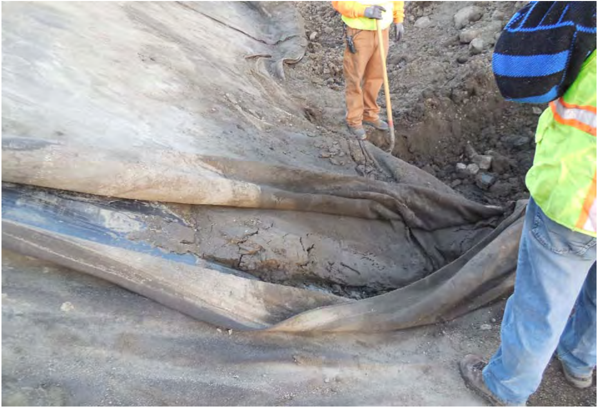
Photo 5 - Fine-grained soils were observed under the geotextile.
