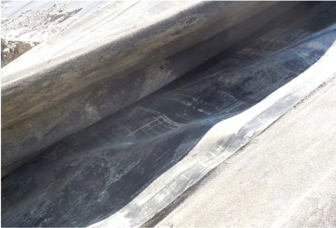
Photo 7 - The liner surface was inspected to confirm that the liner was undamaged.
