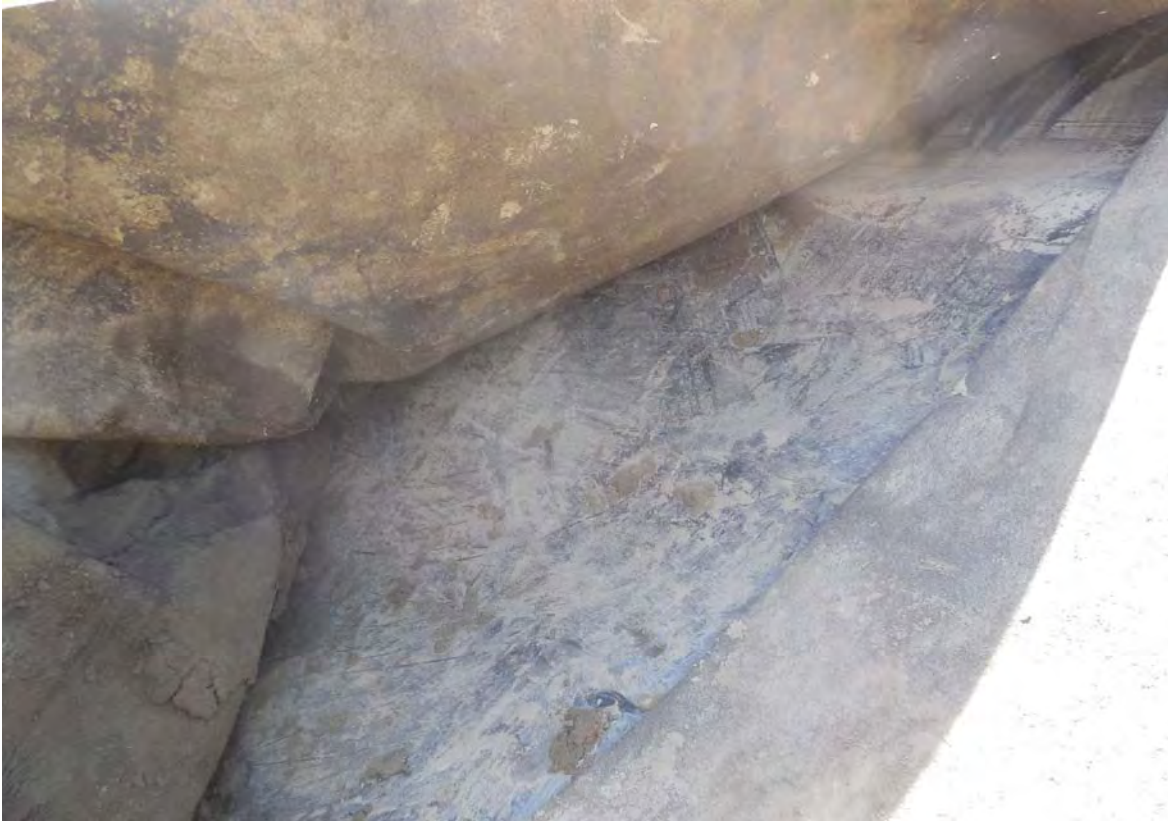
Photo 9 - The liner surface was inspected to confirm that the liner was undamaged.
