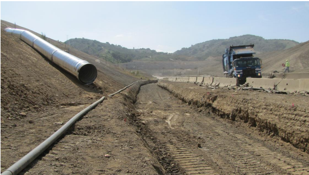
Figure 4 - Grading of New Drainage for Installation of Concrete-Lined Channel Along Haul Road
